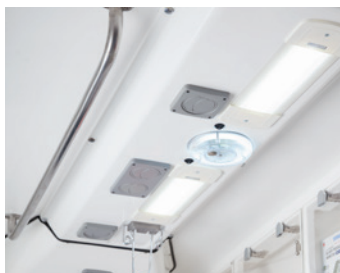
Cabin ceiling services panel
