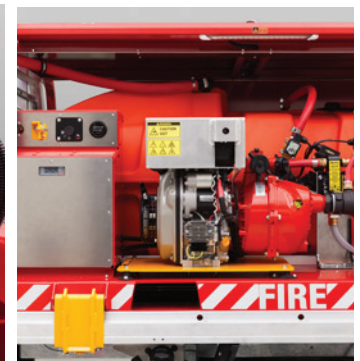
Electric starter kit for davey pump and Pump isolation switch
